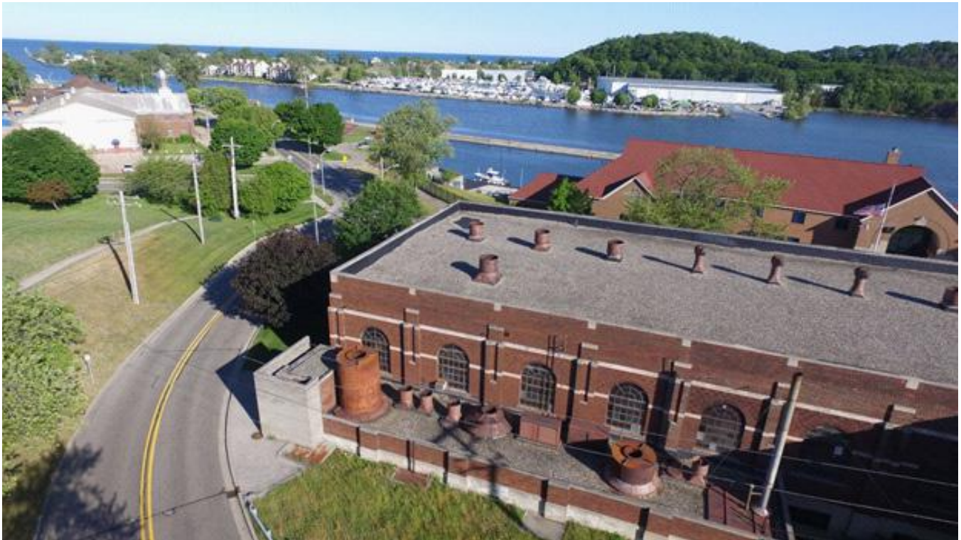
View of western 2/3 of Diesel Plant roof, Coast Guard Station, and the Grand River.
