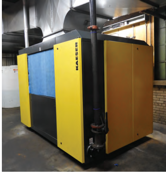
EPC improved its compressed air supply and energy consumption with the installation of a Variable Speed Air Compressor.
