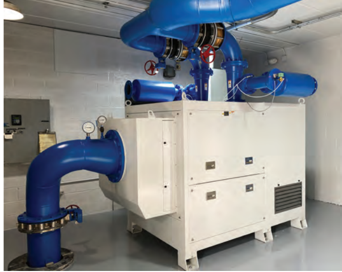
Grand Haven-Spring Lake Sewer Authority replaced two speed motors with energy-efficient dual-core turbo motors controlled by a variable frequency drive.
