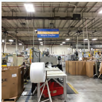
New LED lighting was installed at Cooper Standard in their manufacturing plant and parking lot.
