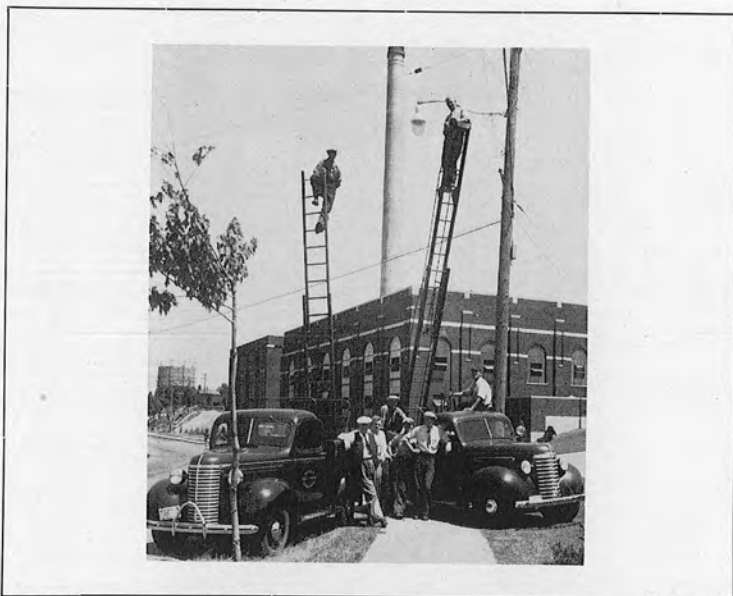
LINE CREW WITH TWO NEW TRUCKS AND EQUIPMENT. POWER PLANT IN DISTANCE.
